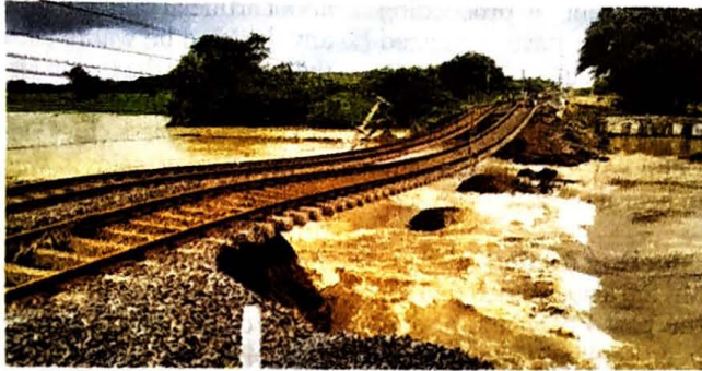
Rain-ravaged: A railway track damaged in the floods at Mahabubabad district of Telangana on Sunday. SPECIAL ARRANGEMENT
